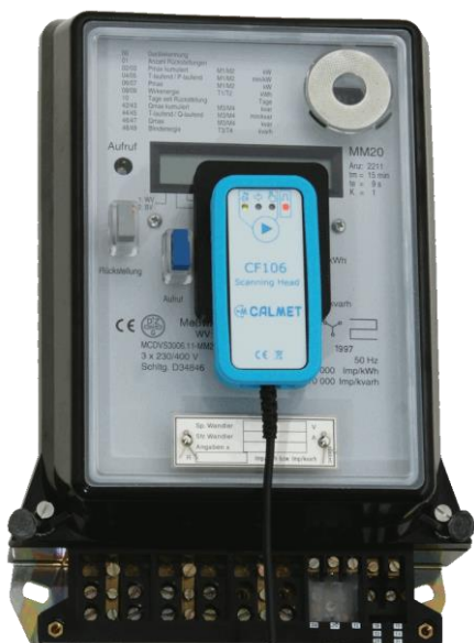
Test of electricity meter with LED (scanning head mounted by self adhesive Velcro)
